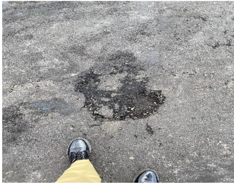
Figure 3 Oil Spillage in Apron
